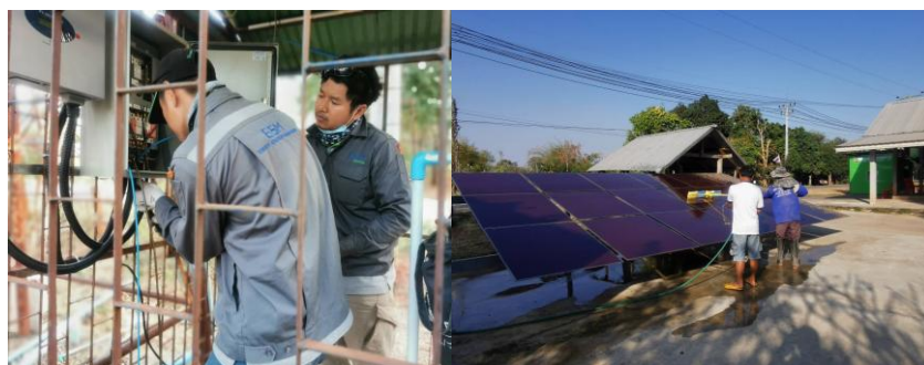
Panels generate electricity for pumping water to supply the village of Wang Udom, Tha Kub Sub-district, Sap Yai District, Chaiyaphum Province.
